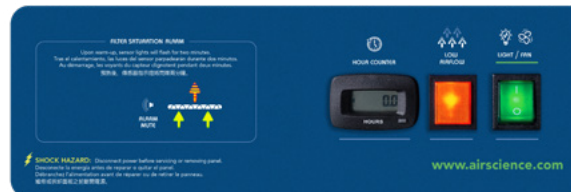
FSA Control Panel
